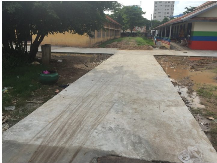
Photo: School renovation 1 building, 5 rooms, 10 classrooms, 1 tiled brick playground with 1 slide, 1 balance, 1 swing, 2 toilets, 2 ramps, 9 trees, 1 rubbish bank, in Toul Kork primary school ,Phnom Penh.
