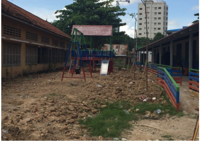
Photo: School renovation 1 building, 5 rooms, 10 classrooms, 1 tiled brick playground with 1 slide, 1 balance, 1 swing, 2 toilets, 2 ramps, 9 trees, 1 rubbish bank, in Toul Kork primary school ,Phnom Penh.
